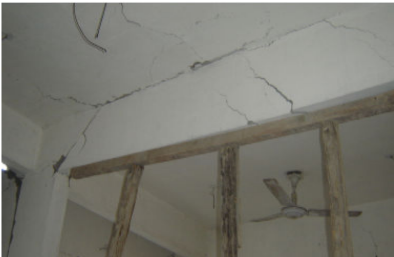
Picture: Damages on beam due to earthquake
