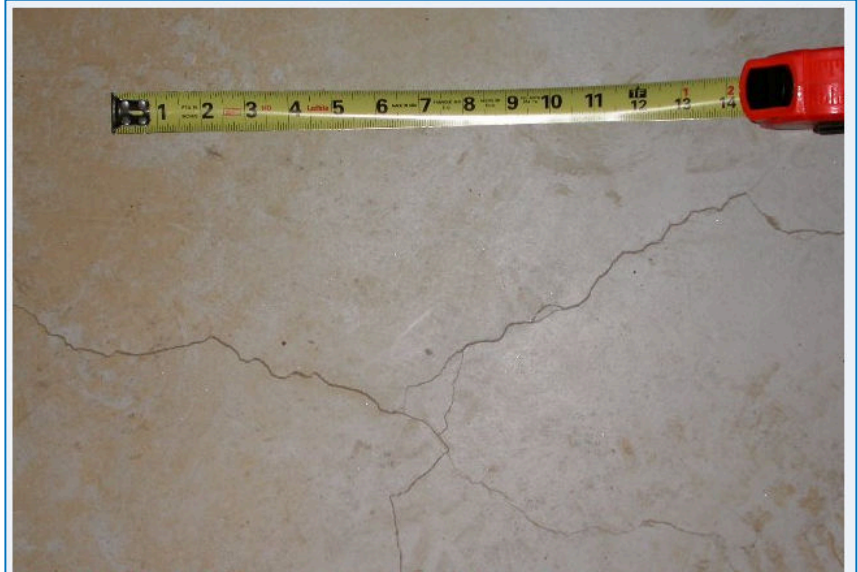
F.1 Minor cracks on floors of ground floor
